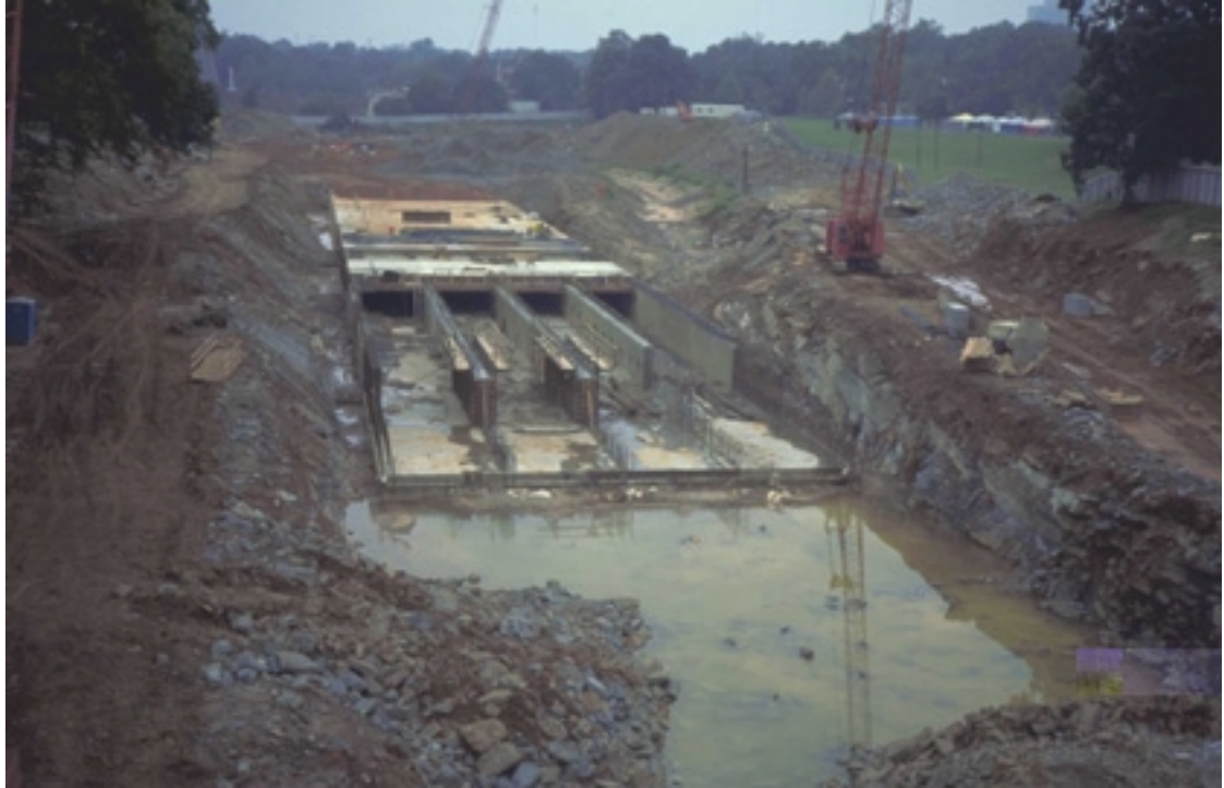
Figure 27: One of Atlanta's Stormwater Treatment Plants
