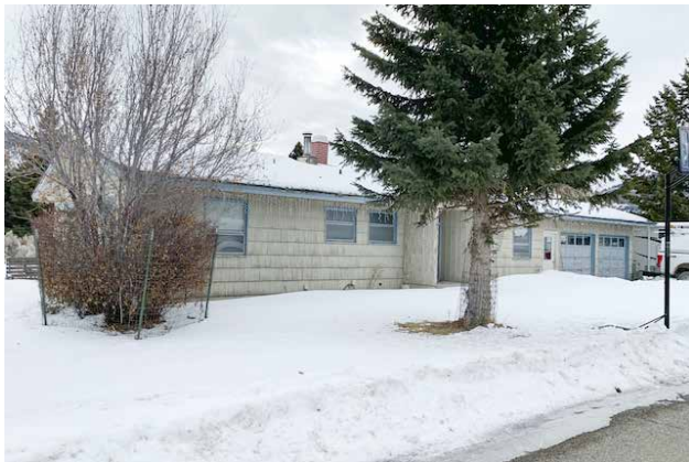
The aging siding on this employee housing in Yellowstone National Park is an example of national park maintenance needs. But why does Yellowstone even have employee housing when at least four gateway communities around the park have private landowners who would be glad to rent housing to park employees? National Park Service photo.
