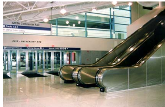
ESCALATOR AT THE NEW ROUTE 128 STATION
